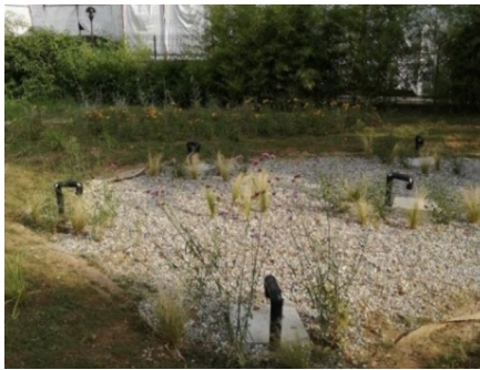
Rain garden to recover rainwater from the roof of the adjacent school.
