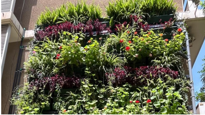
The living walls treating greywater, designed by Iridra in collaboration with American University of Beirut (AUB) and implemented during the Nawamed project in Spring 2023 in Beirut. Image Credit: [IRIDRA], [2024], Used with permission
