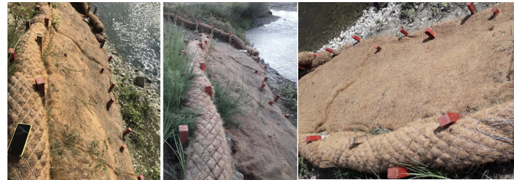
Coconut Erosion Control Blankets (and coir-logs), Erzeni River, Albania, BRIGAD Project. Image Credit: [Eriona Canga], [2019]. Used with permission.
