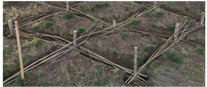
Wattle fencing under construction for upper soil layer retainment. At dry hillside locations, the fence needs to be integrated below soil surface, backfill remains to be done here; Groß Enzersdorf (A).
