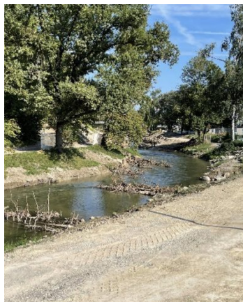
Low cost root wad groynes, River Glatt (under construction), Örlekon (CH) Image Credit: [Rosemaria Stangl], [2023]. Used with permission.
