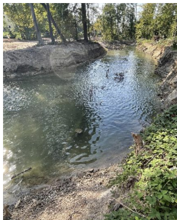
Nature-based low (submerged) and mid-water (semi-submerged) groynes, River Glatt (under construction), Örlekon (CH) Image Credit: [Rosemaria Stangl], [2023]. Used with permission.
